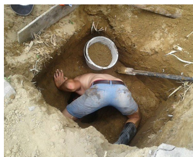
The footings were deep — they went all the way down to the bottom
